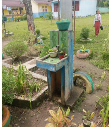
Figure 2. Condition of the Early School Sink
